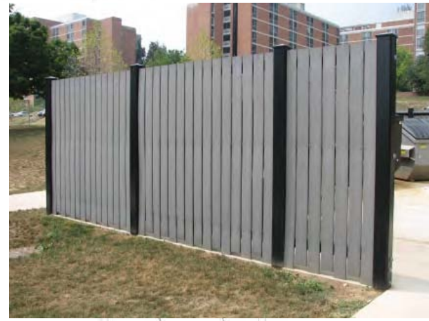
Screen fence fabricated from painted steel tube posts, and frame with recycled lumber planks.
