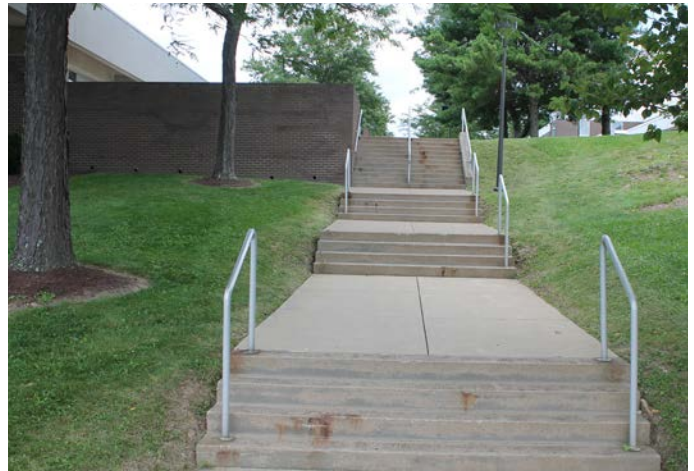
Rust-stained steps early indicator of deterioration
