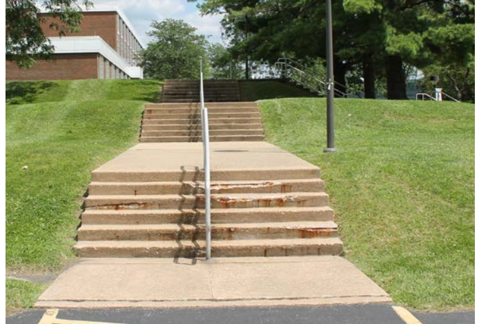
The corners of the concrete steps are chipping away, creating a major tripping hazard
