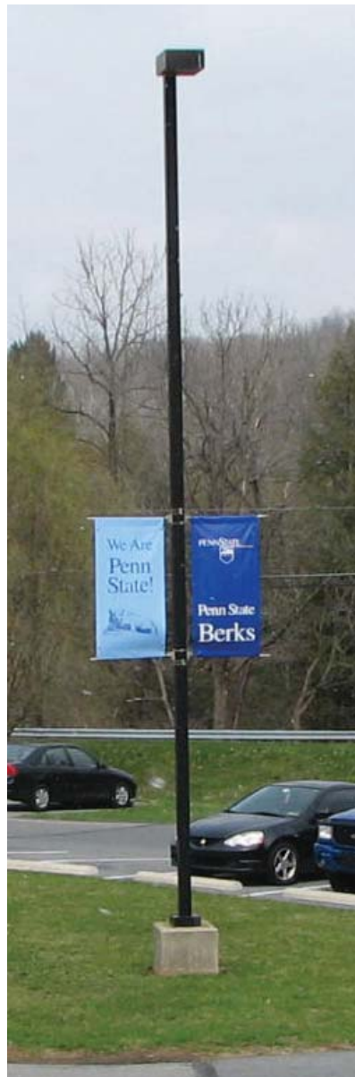
Parking Lot/Roadway Light
